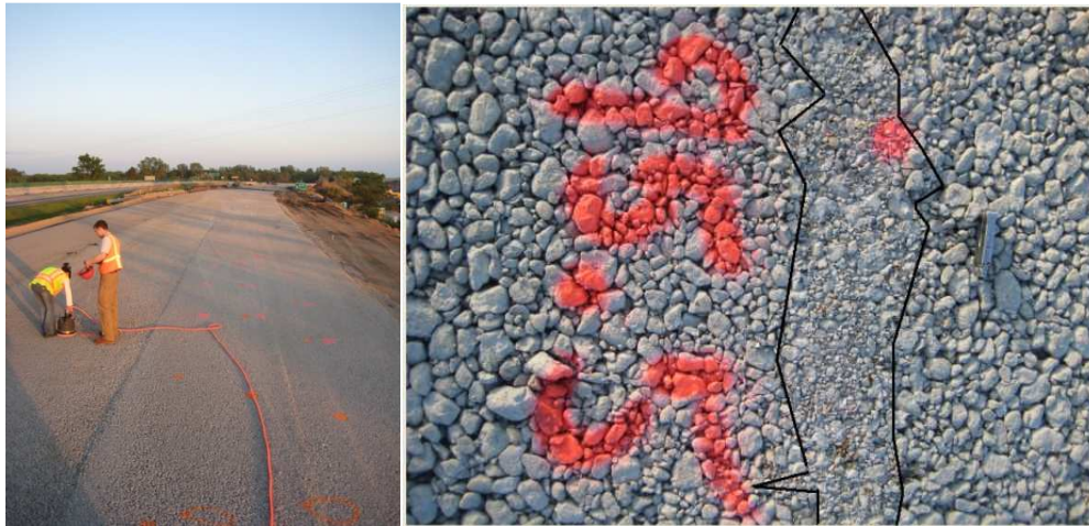
Figure 35. GPT on cement treated base (left) and segregation of CTB on I-96, Michigan.
