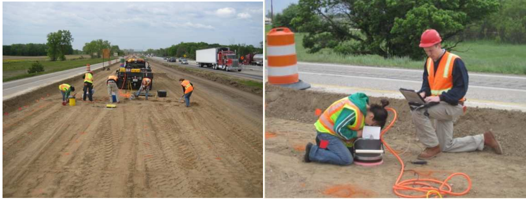
Figure 34. Overview for sandy subbase test bed (left) and GPT in situ testing on I-96, Michigan.
